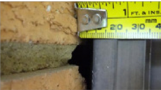
Figure 9 A gap on the external wall surface between frame and brickwork.
