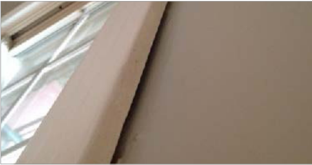
Figure 8 An internal gap between the architrave wall.
