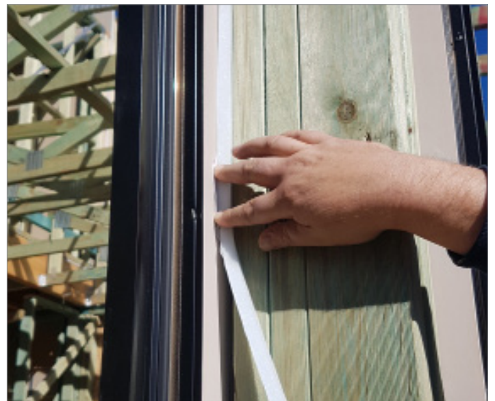
Figure 12 Applying high density acoustic foam to the exterior of the window frame.
